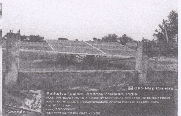
Solar panel for bore well and street lights
