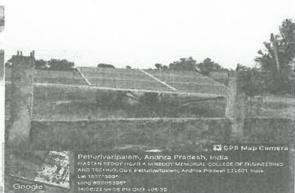
Solar panel for bore well and street lights
