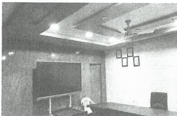
LED bulbs at the board room
