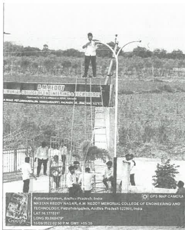
Electronics & Communication Engineering Students Fixing LED bulb to Electric Poles during Project Expo on 15 th September 2022.
